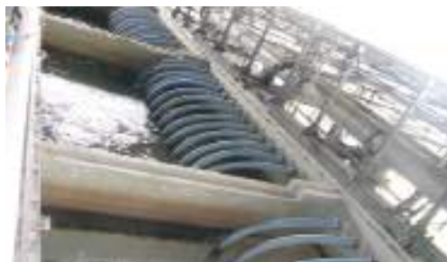
PUB Waste Water Recycling Treatment Plant Singapore
