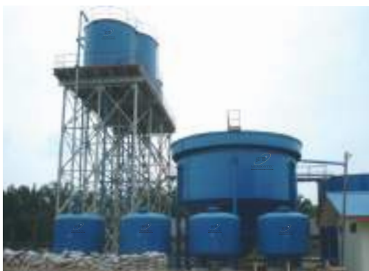
River Water Clarifier System
