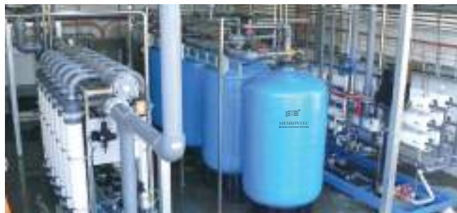
Waste Recycling System (UF+RO+UV)
