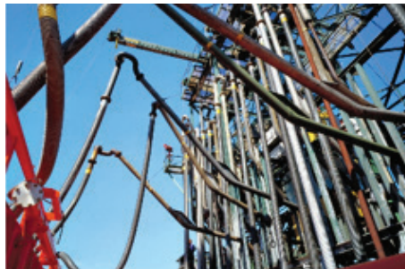
Hoses for oil terminal
